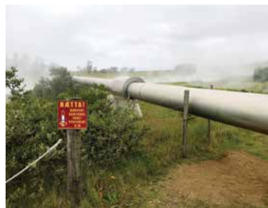
Pipes transport geothermal energy across the island nation.
